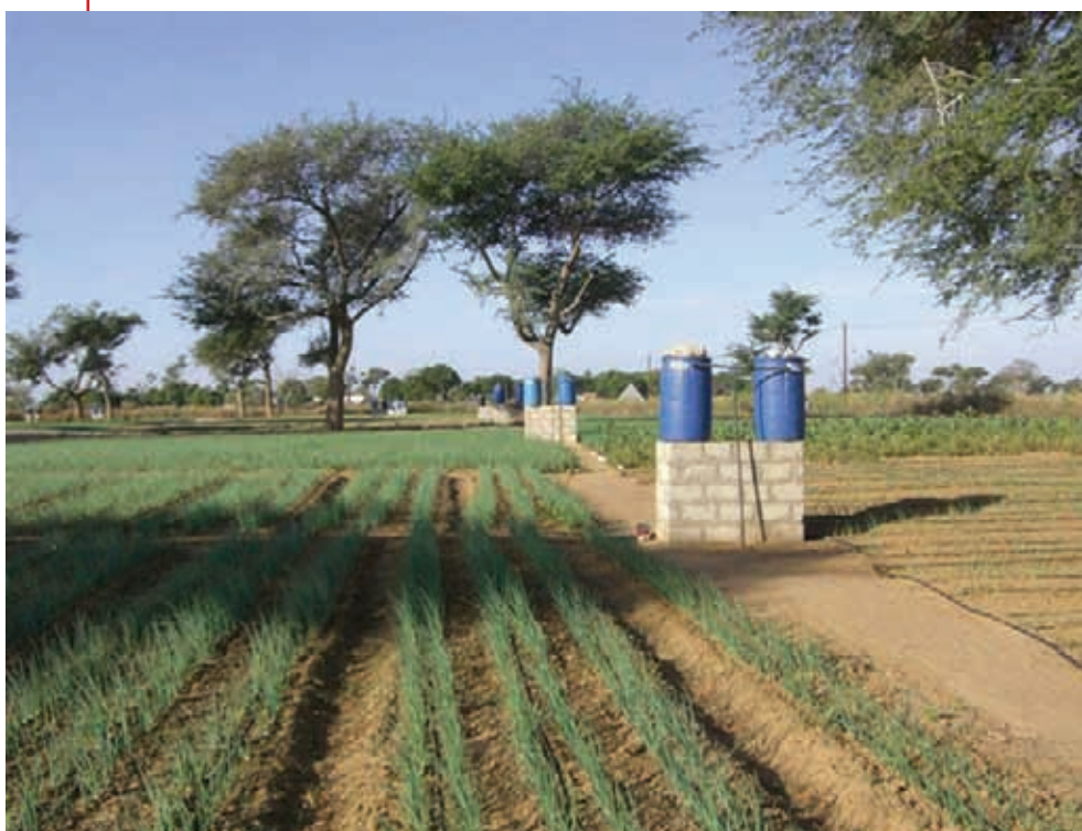
The AMG with the drip irrigation system in place
