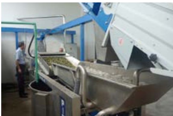
The innovative technologies applied at the plant efficiently utilize inputs and reduce waste while maximizing the quality and quantity of the olive oil.
